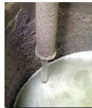
Clear, treated water arrives in the filtrate tank, where it is subsequently routed to a larger filtrate holding tank for reuse or to the sewer.
